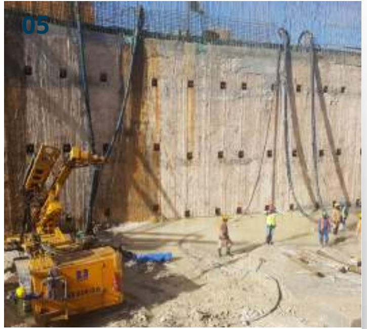
05 Duba ISCC Green Power Plant Saudi Arabia, 2017 Client: Al Saad General Contractor
